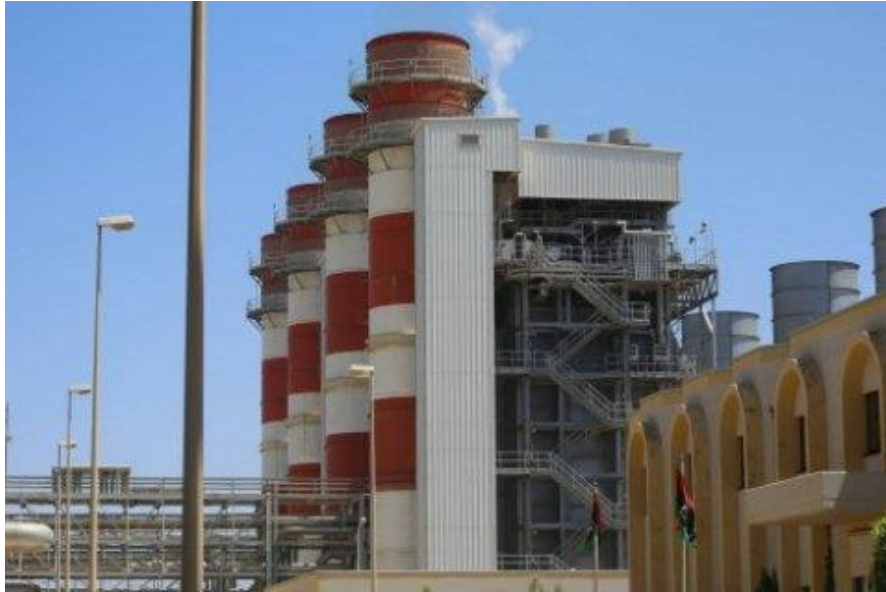
Fig. (2). Picture of the Zawia Combined Cycle Power Plant (ZCCPP)
